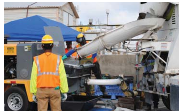
A cement truck begins the initial pouring of grout into Tank 16 at the Savannah River Site (SRS) on June 2, 2015. It was the fifth tank closed since 2012 by Savannah River Remediation, the liquid waste contractor at SRS.
